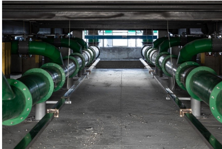
Figure 3. Under pot ducting.
