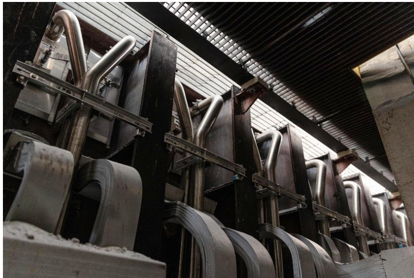
Figure 2. Sidewall mounted SHE units and connection pipes.
