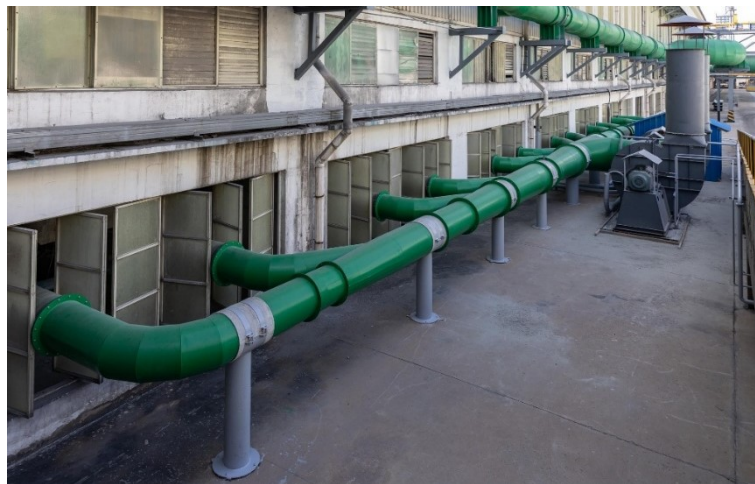
Figure 4. External ducting and fans.
